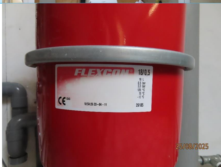
Installaties (G-W-E) (expansievat)
