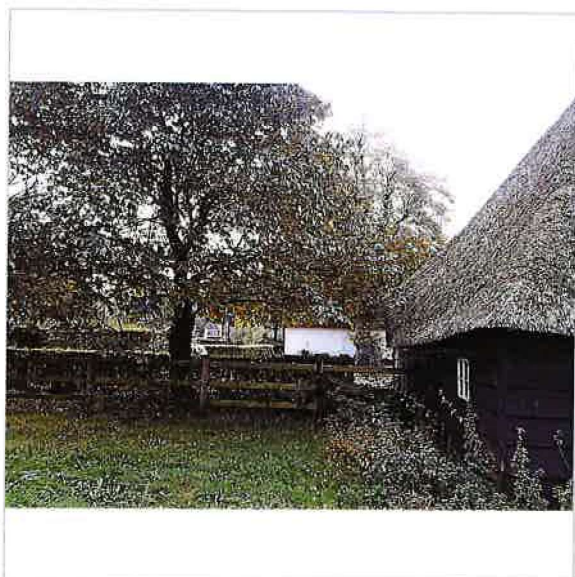
overhellende takken dak no. 4 (foto 2020)
