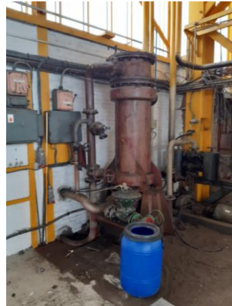
Location bfoto3, inside drum with oil, staining and pipes going outside
