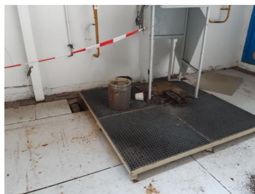
Location bfoto2, metal like staining and clinker in concrete
