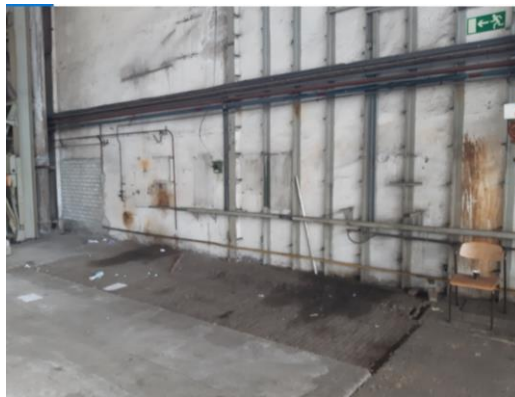
Location bfoto1, oil staining on clinker pavement
