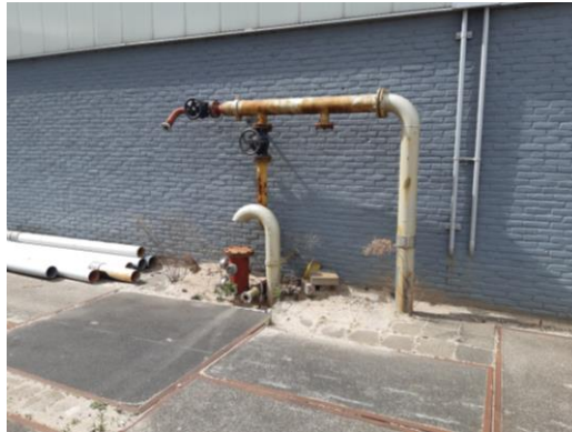
Location bfoto3, pipes through wall outside
