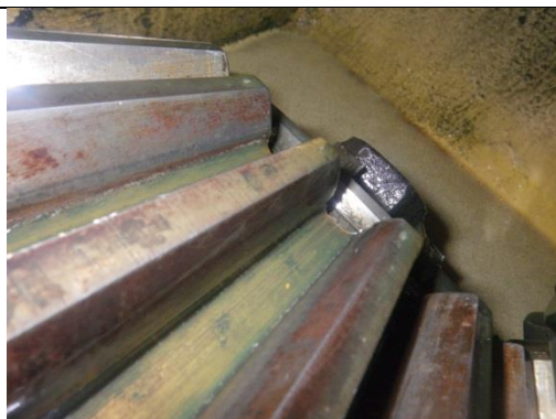
Detailfoto 9: Schade tandwiel inkomende as HTK 1
