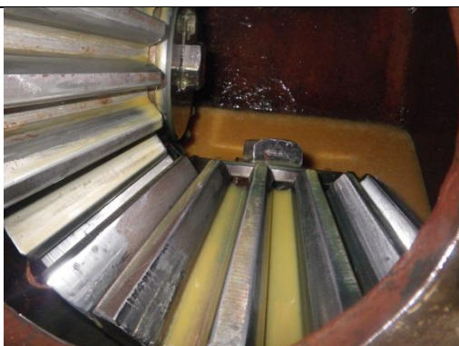
Detailfoto 7: Schade tandwiel inkomende as HTK 4
