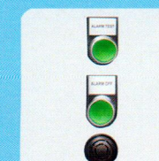
audible & visual leakage alarm
