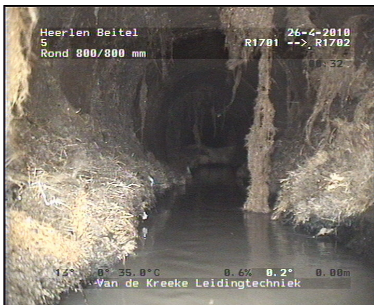
Wortelvorming in riolering
