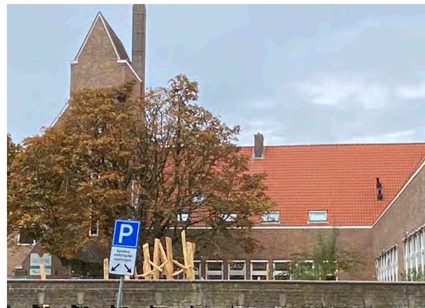
Dakramen: 'opening in pannen', los van dakrand.
