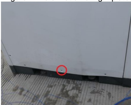
Figure26 Deformation and bolt removing of left plate
