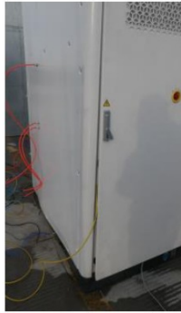
Figure22 Gap of door after explosion
