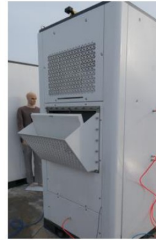
Figure23 Venting panel open as expected
