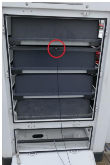
Figure32 Pressure sensor of venting panel
