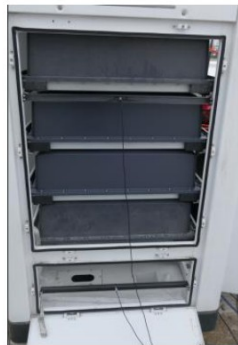
Figure17 Pressure sensors of back-plate side
