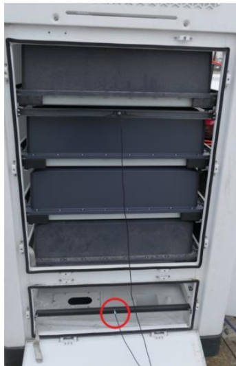
Figure31 Pressure sensor of distribution box
