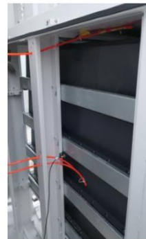
Figure18 Sampling hose of gas detectors
