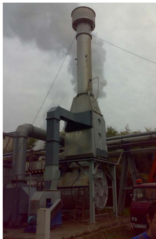
Fig. 5. Data sampling – tested thermal deodorising oxidiser
