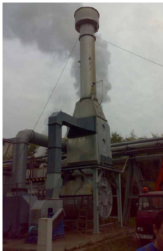
Fig. 5. Data sampling – tested thermal deodorising oxidiser
