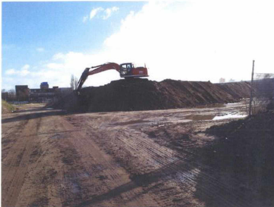
MVB20002 TOP Keileweg Depot Depot 2AO WON - 001
