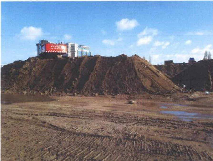
MVB20002 TOP Keileweg Depot Depot 2AO WON - 002
